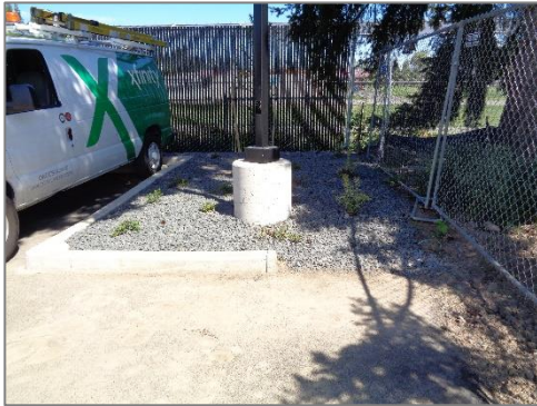
C2-N: North short, broken curb
