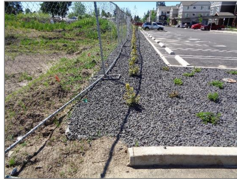
C2-S: South short, broken curb
