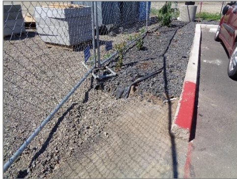
C1b: West broken curb
