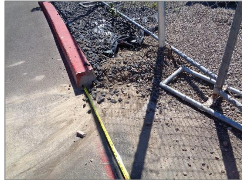
C1c: East broken curb
