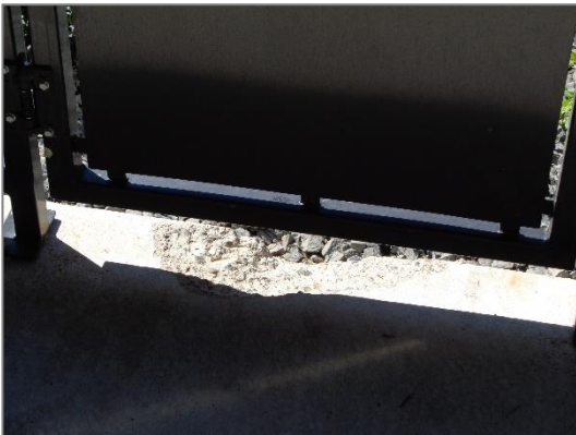
D: Apt. B103 gouged concrete under patio gate
