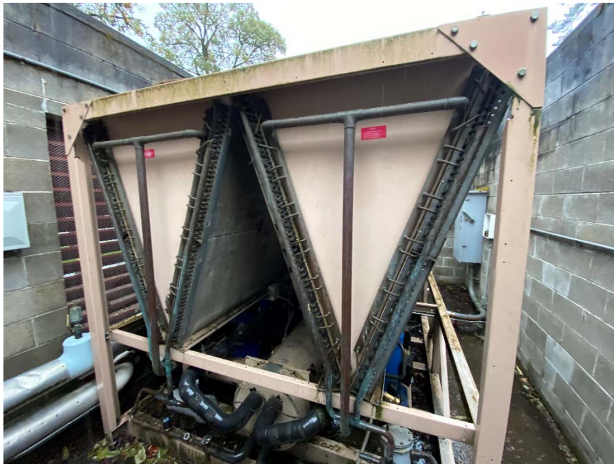
Figure 33: Chiller (CH-1) – Outside of Mechanical Room Entrance
