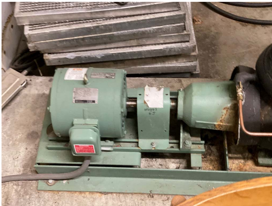
Figure 31: Chilled Water Pump (P-1) - New Library Mechanical Room
