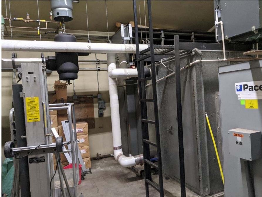
Figure 28: SF-1 & CC-1 - New Library Mechanical Room
