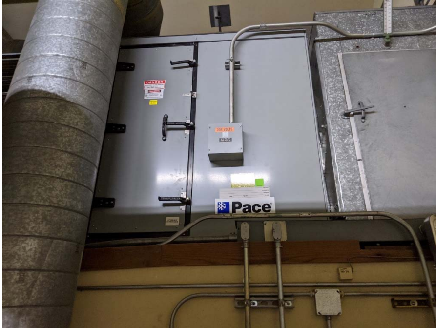
Figure 32: Return Fan (RF-1) New Library Mechanical Room
